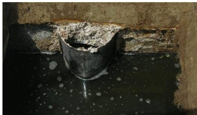
Photo 1 Concrete Corrosion around Outlet Baffle
